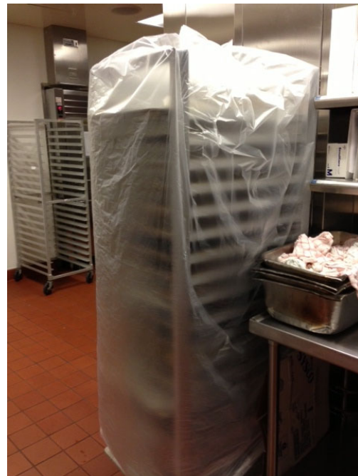
Covered clean equipment not in use
