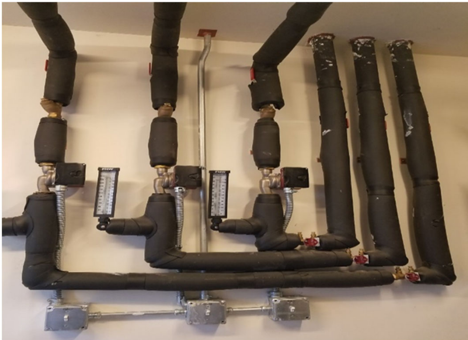
Hot water for distribution
