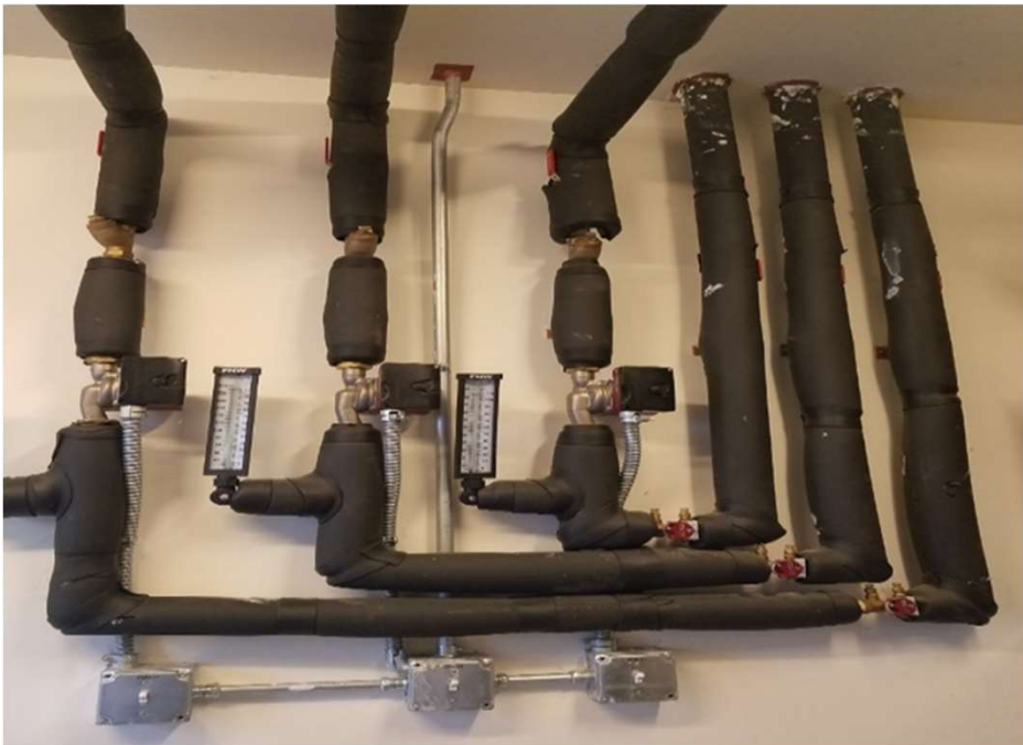
Hot water for distribution
