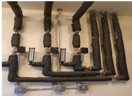
Hot water for distribution
