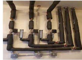
Hot water for distribution
