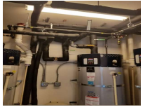
Recirculating hot water heaters in series
