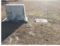
Water meter and backflow prevention device
